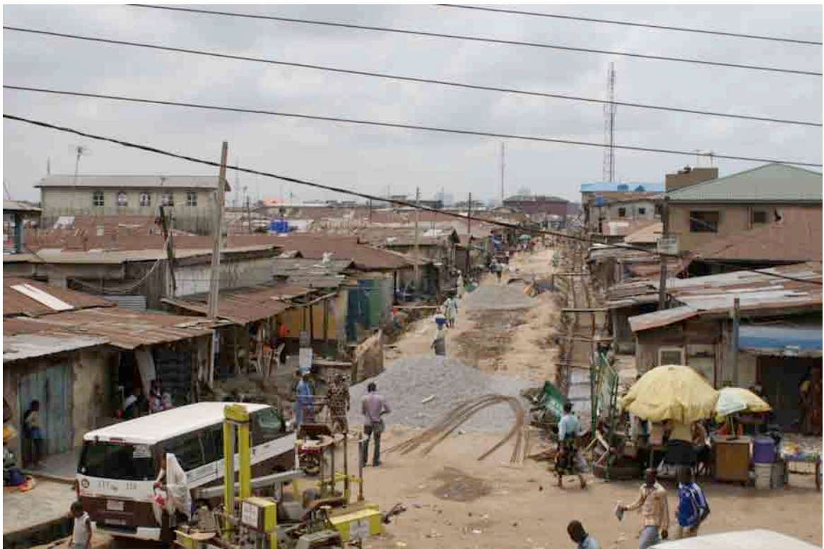
Figure 7.16: A ROAD CONSTRUCTION THROUGH AN EXISTING BUILT-UP AREA (Photograph by Olusegun Oluwole).
