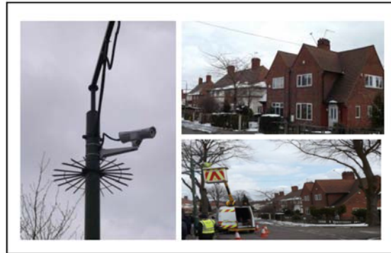
Figure 1: The installation process of the autonomous infrared camera
