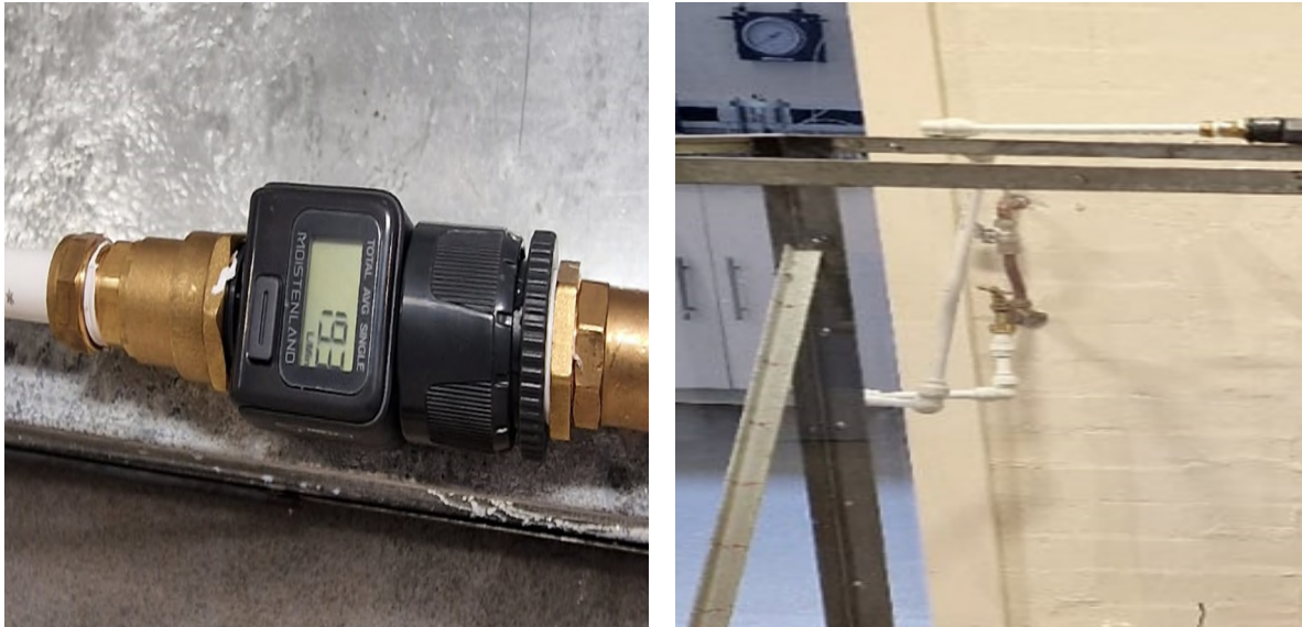
Figure 3.9: Main water supply valve (left) and flow meter (right) to record the water flow rate
