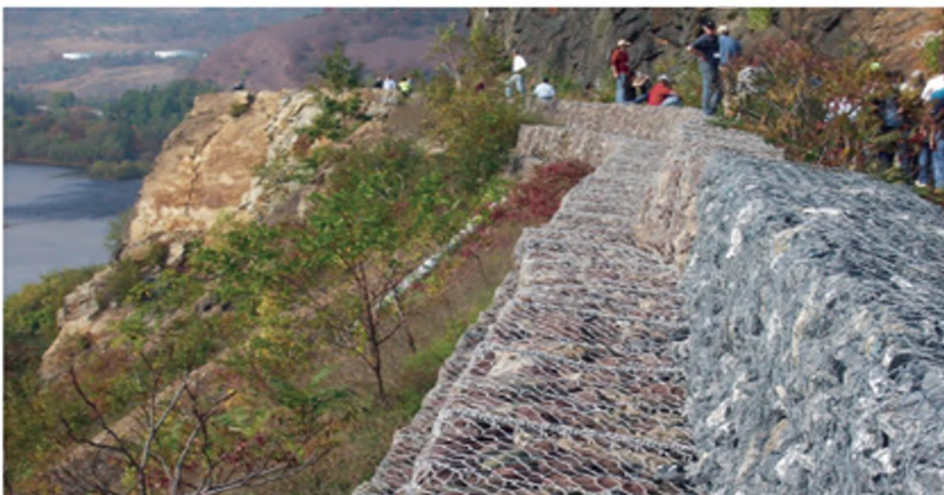
Figure 2.8: Schematic and photograph of a gabion wall along a highway. (Photograph of gabions located in the Pocono Mountains, Pennsylvania, USA, by Lynn Highland, U.S. Geological Survey.)(Highland and Bobrowsky, 2008)
