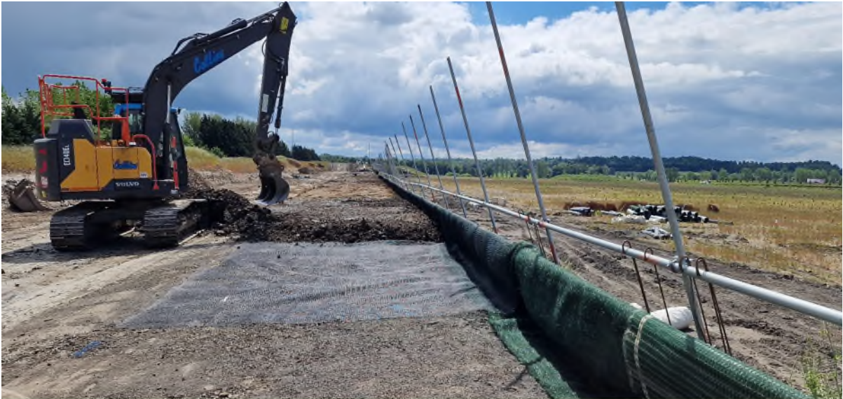
Figure 2.14: Installation of Geo-synthetic textile to stabilise slope at Northampton Gateway Site Project (Reference: image taken by the Author during site visit in June 2024)
