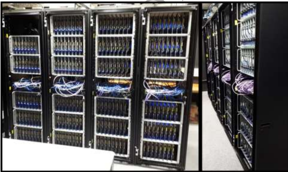
Fig. 2: Front and side view of the HPC FPGA cluster
