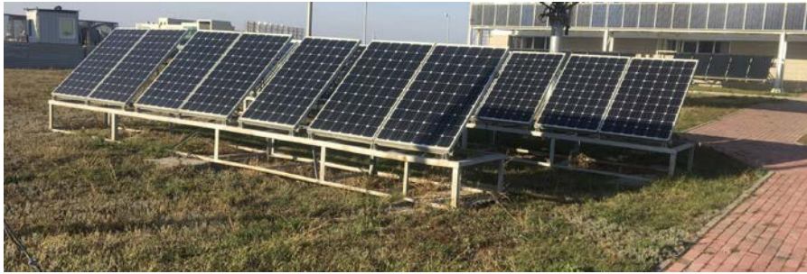
Figure 2. PV solar panels connected to the “Yurt” building
