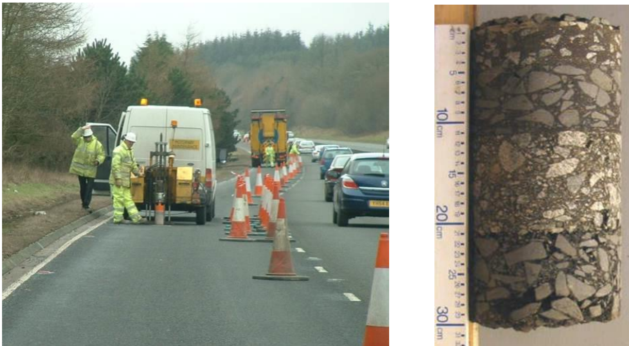
Figure 2. Coring rig extracting asphalt (left), and 300mm thick asphalt core taken from pavement (right)
