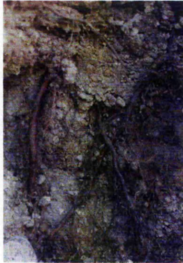
Figure 2.4. Exposed roots in an investigation trench observed to be exploiting fissures in Gault Clay, Longham Wood Cutting, CIRIA bioengineering trial (Greenwood et al. , 2001).
