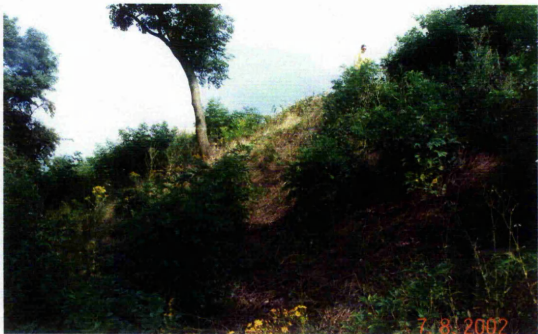
Figure 4.7. View of railway embankment looking north towards Ruddington. Vegetation along the embankment consists of ash and sycamore trees with an understory vegetation cover of elder and hawthorn shrubs, grasses, nettles and brambles (Photograph A. Swift).
