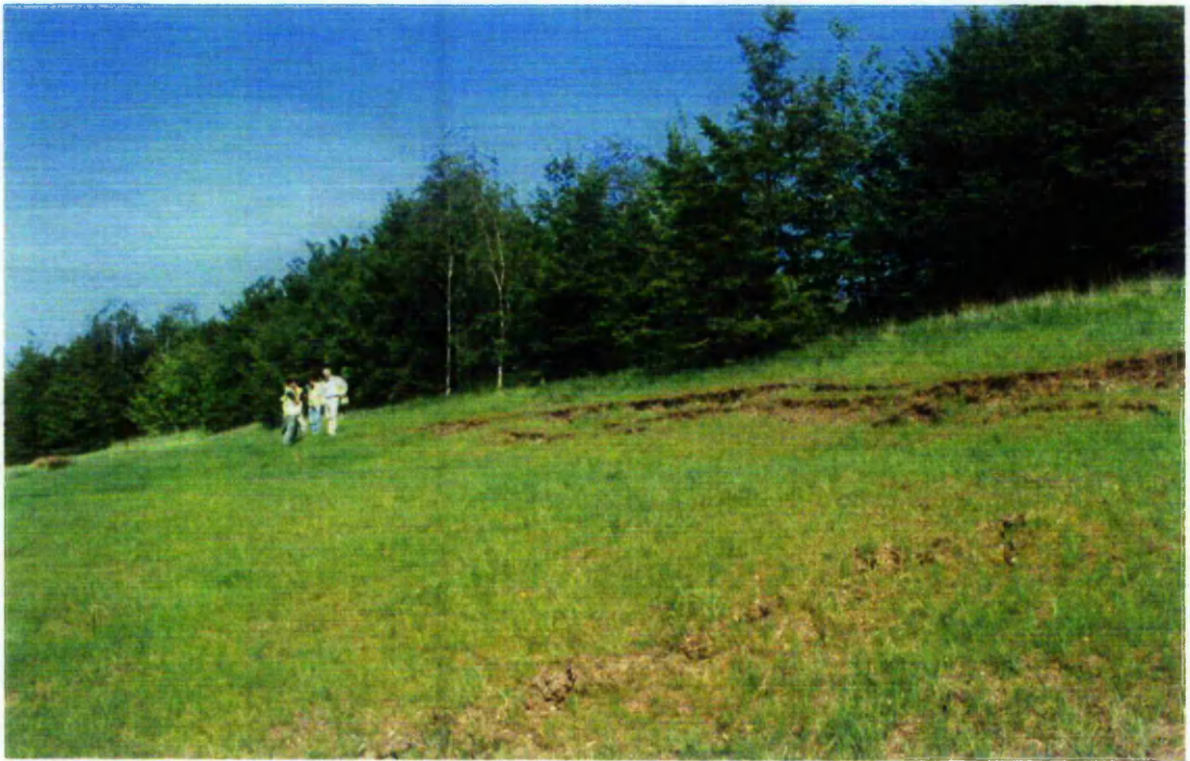
Figure 4.5. Shallow landslide occurring in cutting section adjacent to field site. NB. Tree line is above top of landslide scar, landslide has occurred where there are no deep rooting plants. Taken September 2002.
