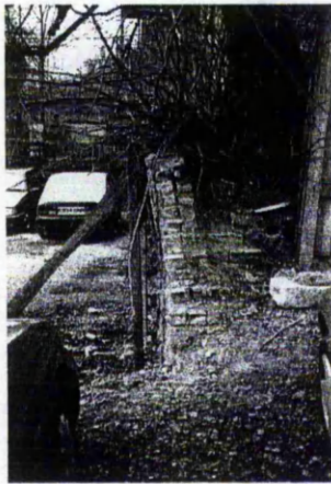
b). Retaining wall damage due to roots at Nottingham Trent University
