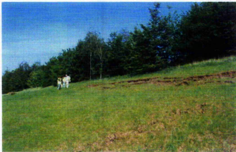
Figure 3. Instability of cutting slopes on the M11 near Loughton. Adjacent vegetated areas appear more stable.
