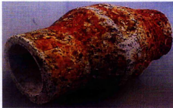
Figure 49. Moulded conduit with internal collapse at one end
