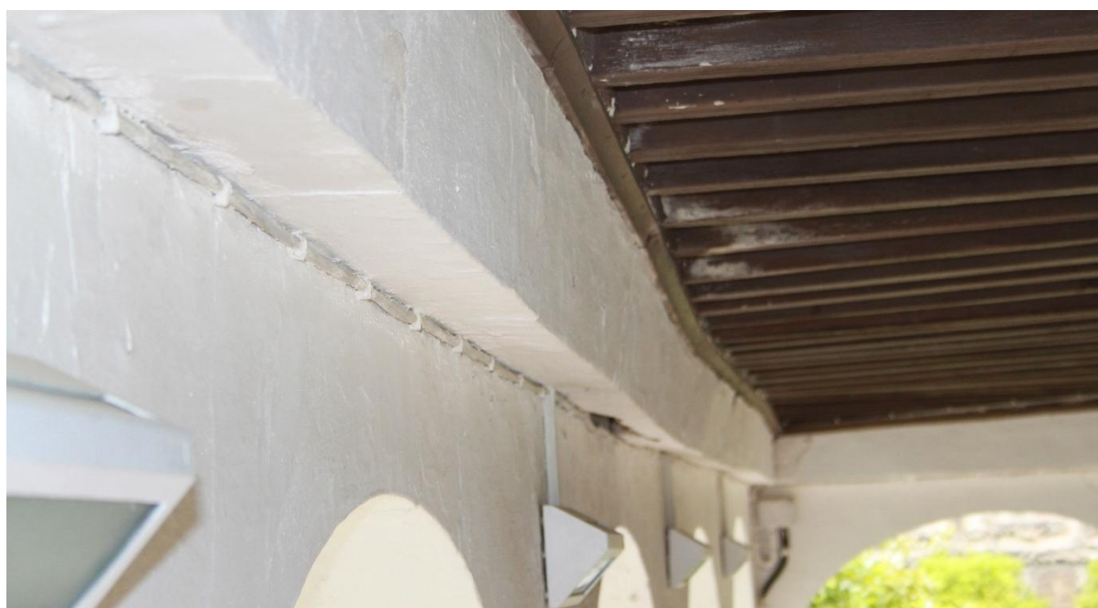
Figure 10. a) TLS point cloud over model without deformations. b) Photograph of the rafters and beam's displacement.
