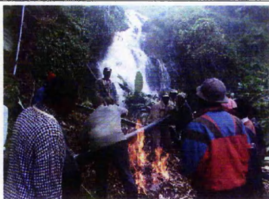
Small bends were made by heating sections and then shaping around a former. Embers rather than flames (as above) should be used to avoid the risk of melting the pipe completely.
