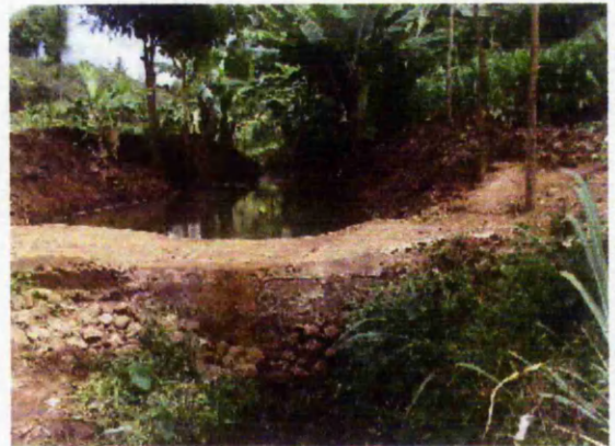
Completed intake with storage pond
