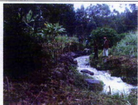
A few hours later, a stone platform has been constructed to support the pipe.
