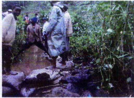
Boulders have been used to form a deep pool around the intake. Soil bags seal the gaps.
