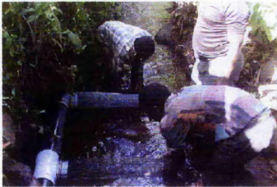
Galvanized wire mesh prevents debris from pool entering the penstock at the intake
