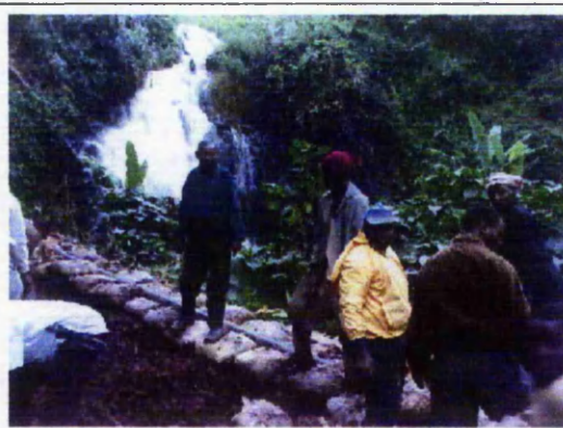
The entire penstock was supported by soil bags wherever possible and covered to prevent damage by sunlight.
