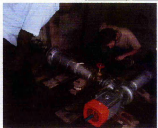
The induction motor as generator produces 2.2kW but a shaft extension provides a 3kW drive for mechanical loads.
