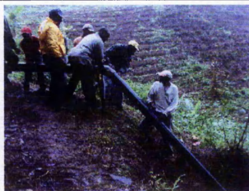
Since PVC is quite rigid, 45° elbows joints were cemented in at two points to enable the penstock to follow the shortest path to the turbine house.
