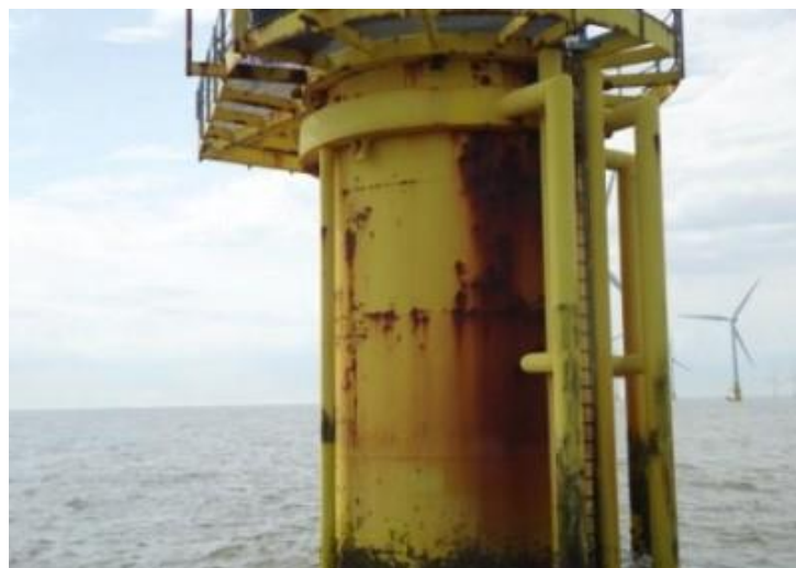
Figure 1.3: Extent of corrosion in splash zone region (ABFAD 2020).
