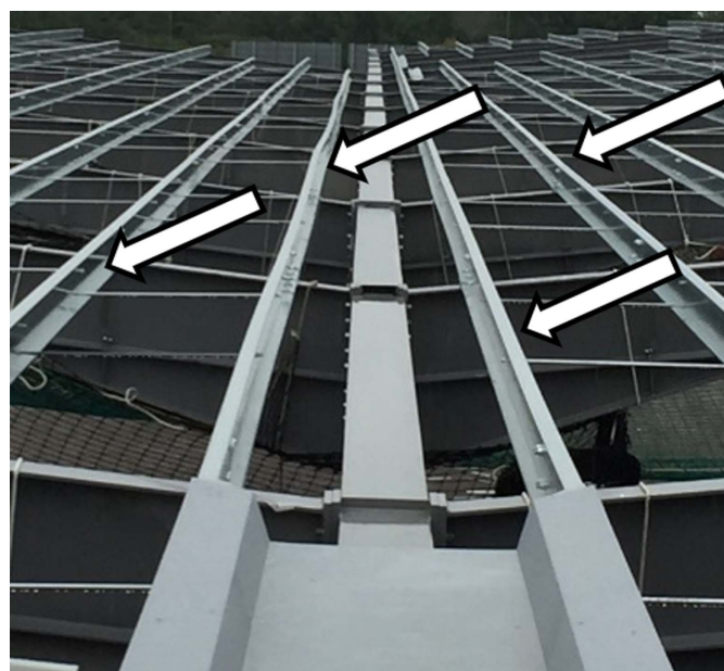
Fig. 8. Wavy purlins on the roof.
