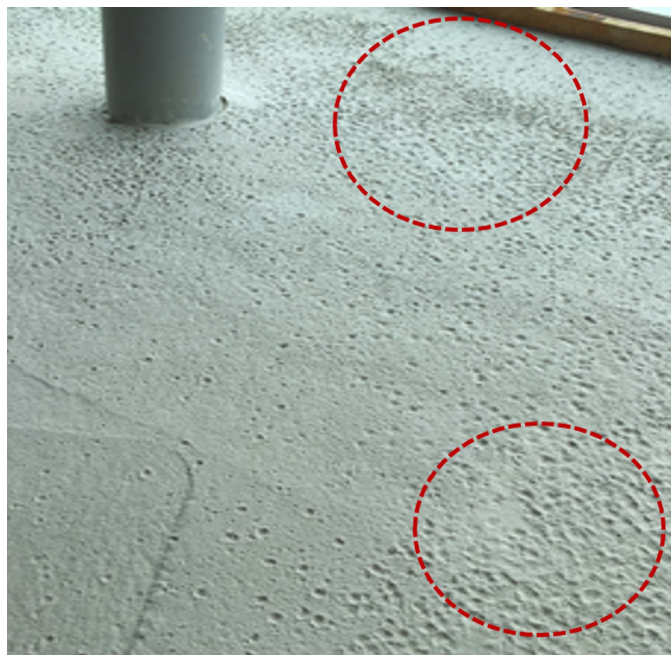
Fig. 2. Flatness of concrete slabs affected by special issues.
