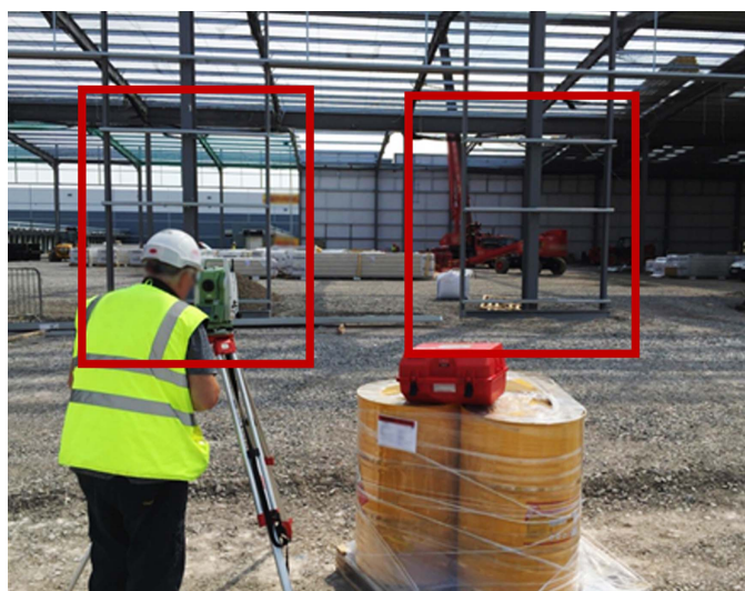
Fig. 7. Misalignment of stanchions.
