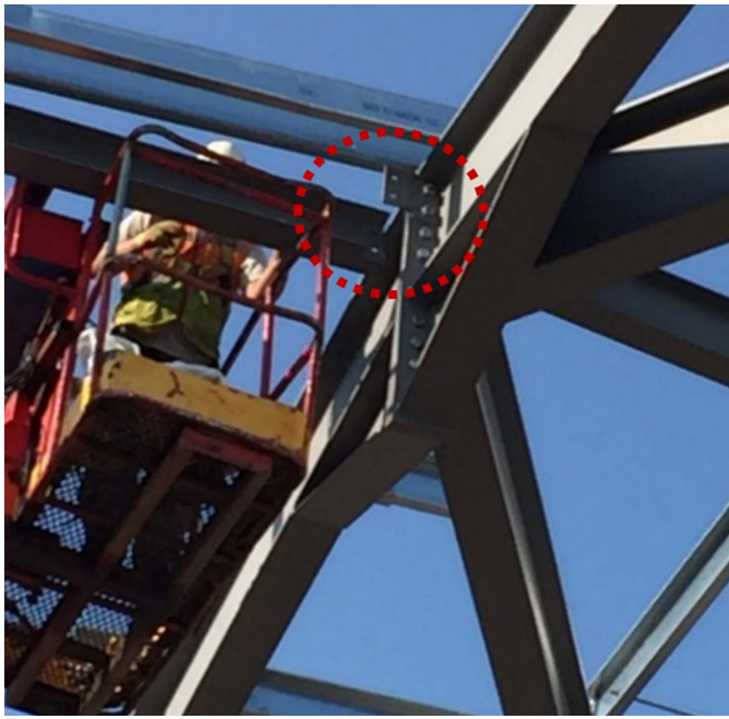
Fig. 9. Lack of fit of the beam between two grid lines.
