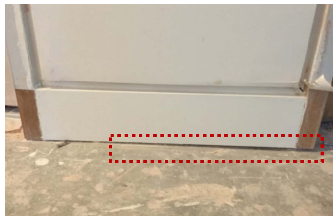
Fig. 1. Excessive gap between the skirting and the concrete slab.
