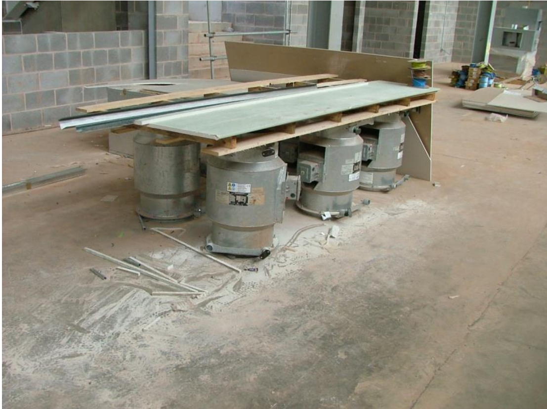
Figure 3: Air-handling units used as a work bench
